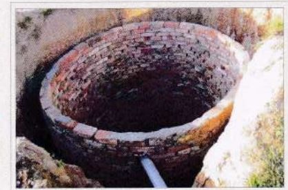
A water soak pit near the rearing house for collection and disposal of water used for cleaning/washing/disinfection from the silkworm rearing house
